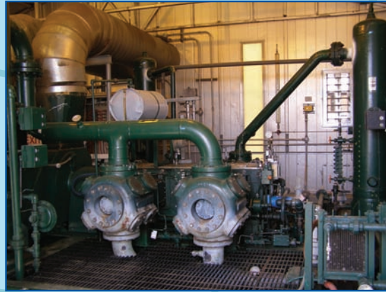
Quickly scan inside compressor buildings, inlet and treater buildings.
