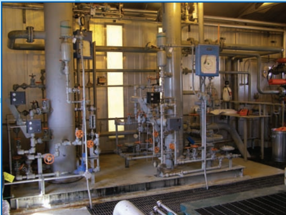
A leak that is in the back of, or behind a component may still be visible to the camera
